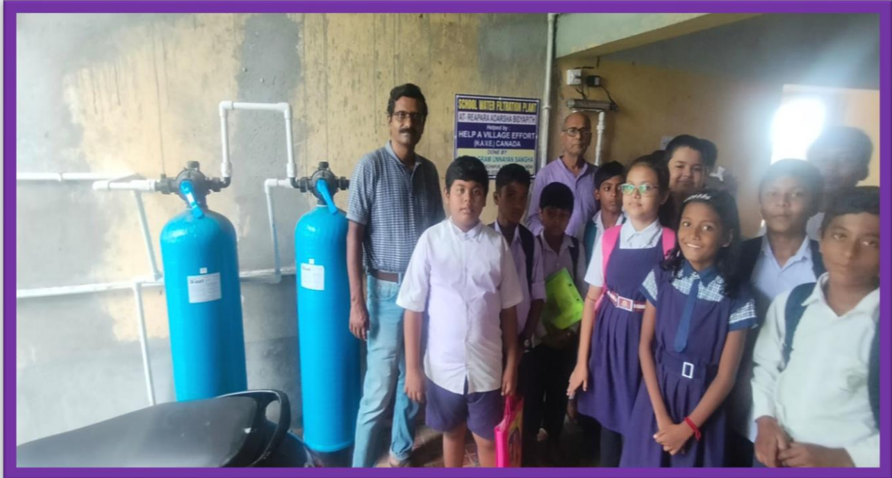
SCHOOL WATER FILTRATION PLANT ( REYAPARA ADARSHA BIDYAPITH)
