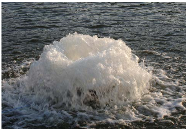
Figure 4 Float-mounted vertical pump aerator in operation
