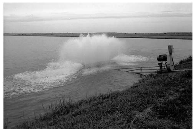
Figure 5 Pump sprayer aerator in operation
