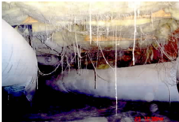
The writer's house: strings of dust were hanging in the crawl space because the house's central vacuum was improperly vented to the basement. This was one of the many items of concern that were not noted in the pre-sale house inspection report.
