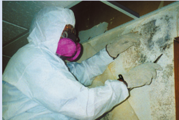
Photo 7: Remediation worker with limited PPE
