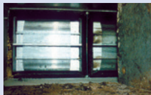
Photo 4C: Moldy air duct
