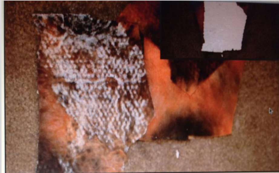
Upper right shows that thick paint that was used to coat the inside of the AC supply plenum. Rather than removing the mold, they simply painted over it. Bottom picture is very heavy mold growth found when the heavy paint was peeled off.
