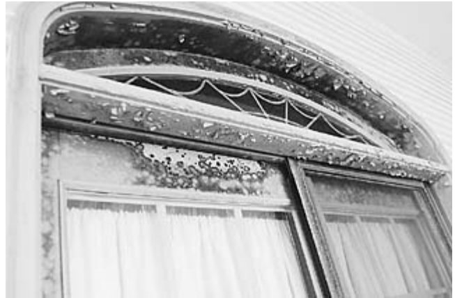
Mold fills a window of Ballard's Dripping Springs mansion. (Photo By Jana Birchum)
