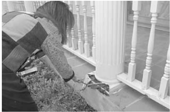
Ballard examines some of the damage done to her home by mold. (Photo By Jana Birchum)
