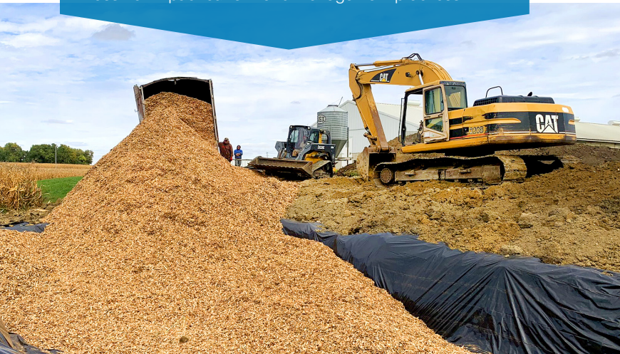
A bioreactor installation. Wood chips form the filter in the system.
