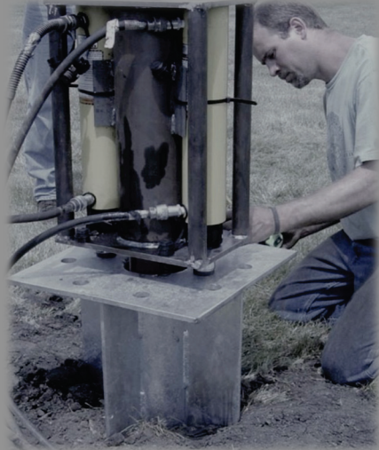
Bearing capacity is precisely calculated upon the hydraulic system's pressure gauge reading and hydraulic cylinder specifications.
