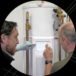
Onsite assisted commissioning
