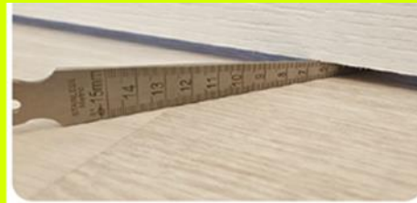
Insufficient ~6 mm internal door undercut identified during verification
