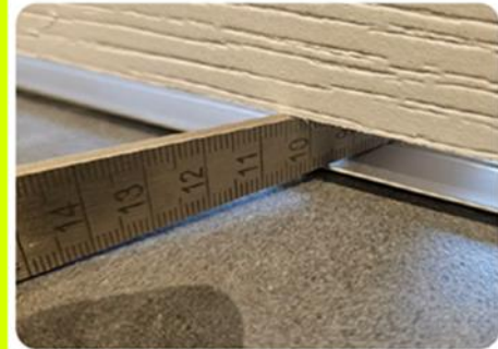
Door undercuts corrected to 10 mm
