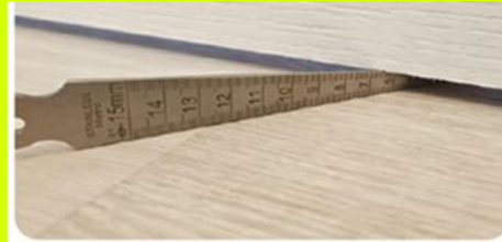
Insufficient ~6 mm internal door undercut identified during verification
