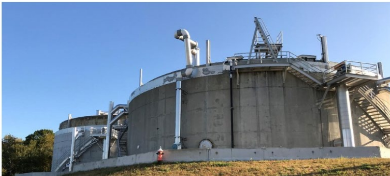
Greater Lawrence Sanitary District Digester
