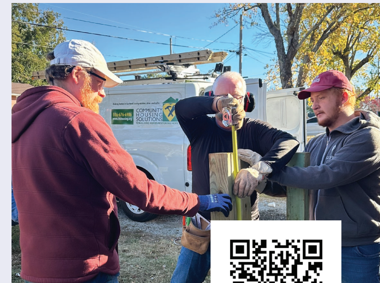
Volunteers from Forest Hills Presbyterian Church work on building handrails on Ms. Pemberton's front porch.
