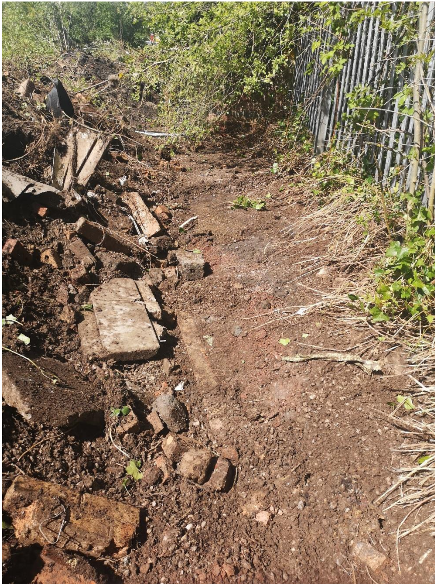
Figure 17 Area below furnaces with demolition debris and length of kerb from car parking area.
