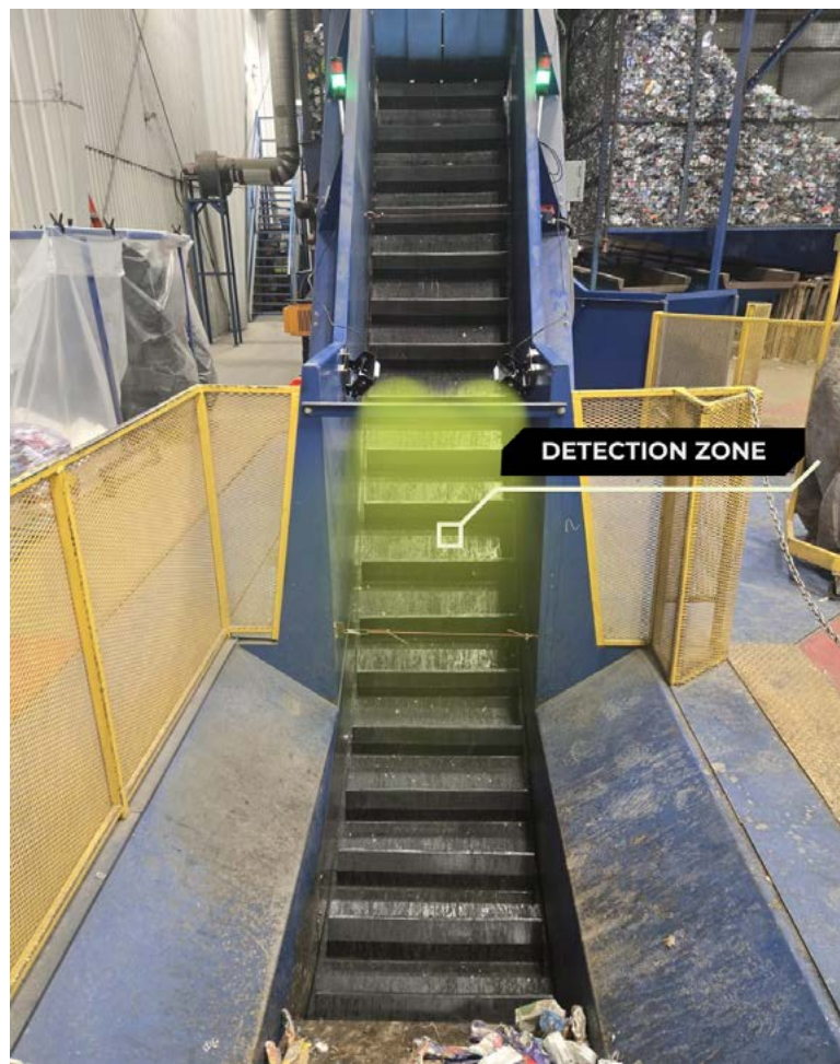
SCAN~LINK installed on a conveyor system.
