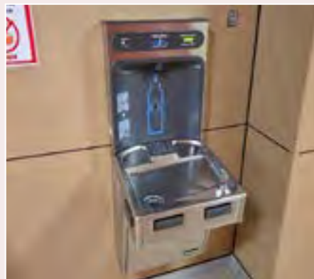
✓ WATER REFILL STATIONS AND FOUNTAINS Completed August 2023
