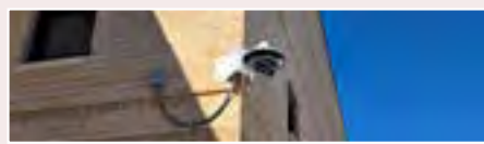
⌚ ACCESS CONTROL AND SECURITY CAMERAS Anticipated completion January 2025
