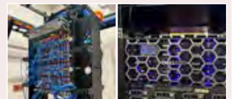
✓ TECHNOLOGY INFRASTRUCTURE Dark fiber project completed June 2024
