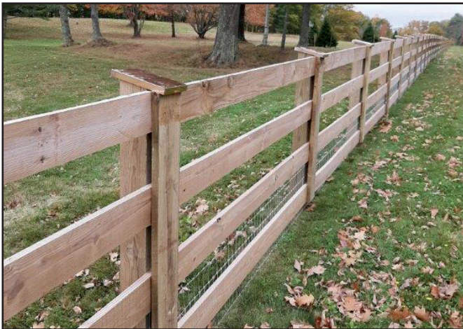
4 BOARD NAIL ON FENCE WITH FACEBOARD AND COPPER CAP PLUS 2"X4" WOVEN WIRE
