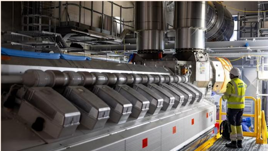
Engines inside Europe’s first data centre microgrid in Dublin. Operator Pure Data Centres says it is a ‘creative solution’ to Ireland’s strained electricity grid © Pure DC
