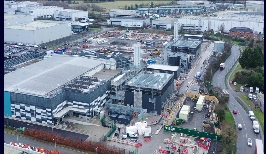
Pure DC deploy Europe's First Data Centre Microgrid
