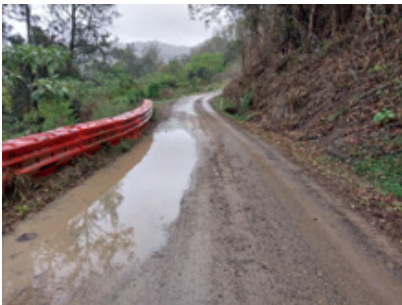
Plate 6.3 Kempsey Road – Road not free draining and slippery conditions
