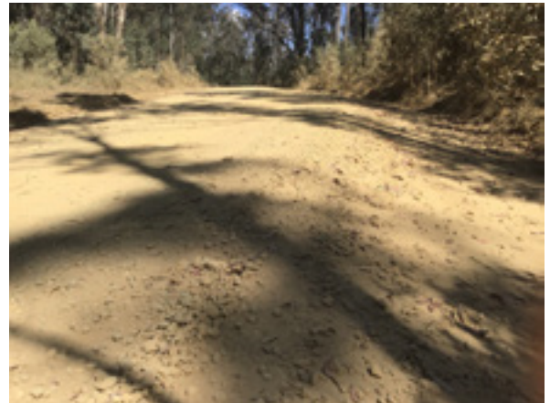
Plate 6.2 Protruding aggregates/ rocks and loose materials – North of Falls Road
