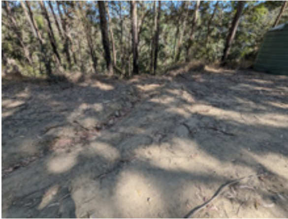
Plate 6.7 Kempsey Road – Road Reserve Soils Western Section – Erosion in Drainage Controls
