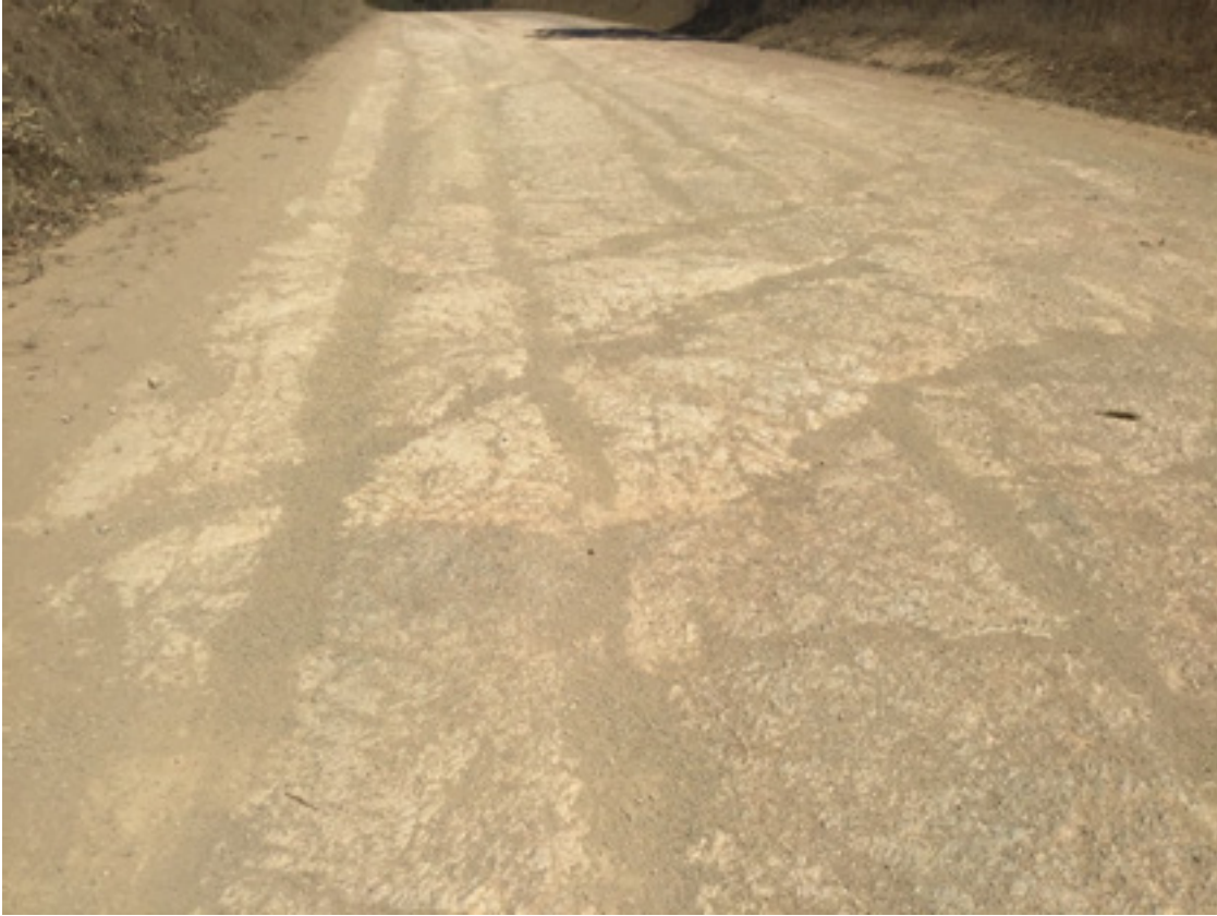
Plate 4.12 Channel erosion and loose materials – East of Five Day Creek
