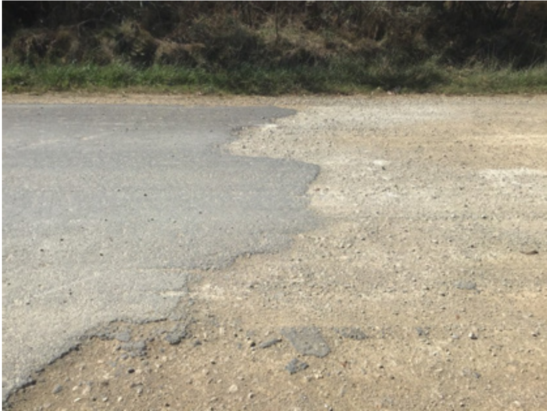
Plate 2.3 Kempsey Road – South of Williams Rd – Seal to Unsealed connecting seam
