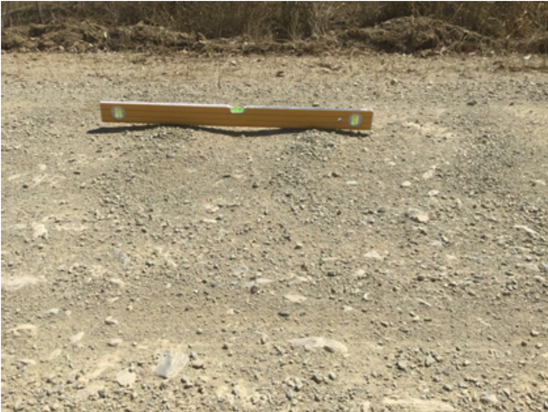
Plate 4.13 Corrugations and protruding aggregates – East of Five Day Creek
