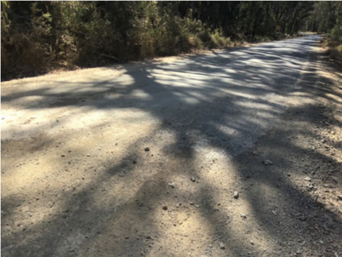
Plate 4.6 Pavement seam with signs of deterioration – South of Styx River Crossing
