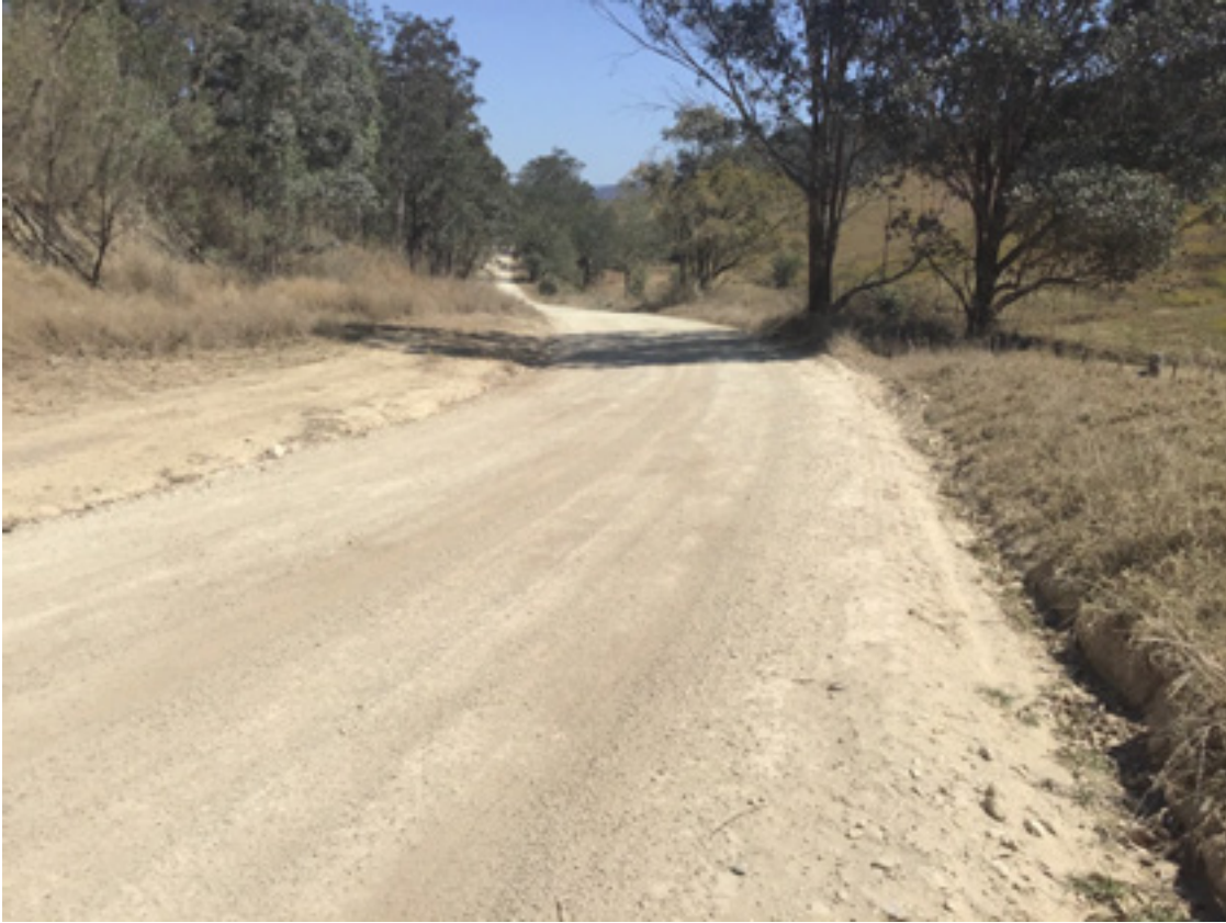
Plate 4.14 Loose material, shoving and rutting – East of Five Day Creek
