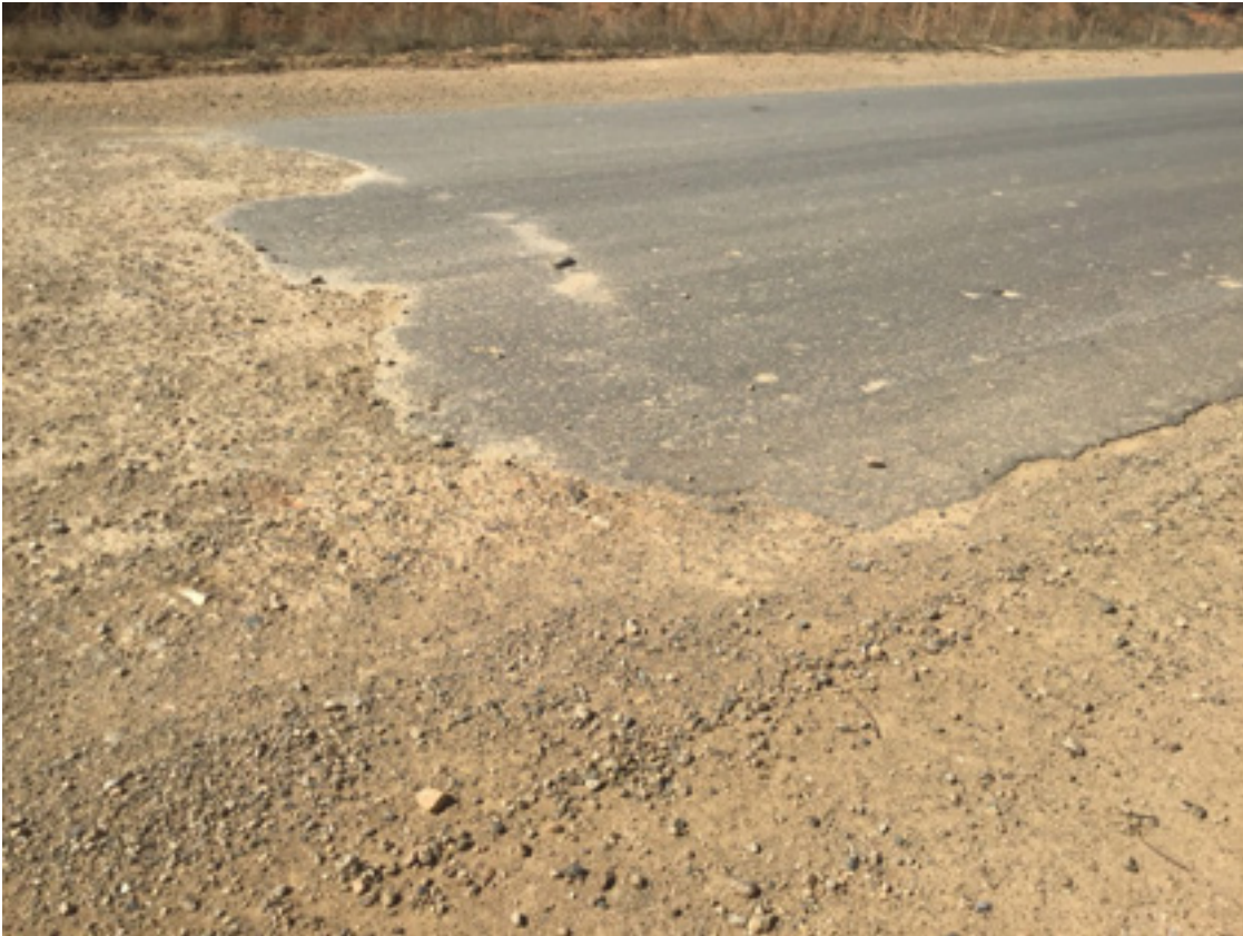
Plate 4.4 Pavement connection seam with signs of deterioration – North of Williams Road
