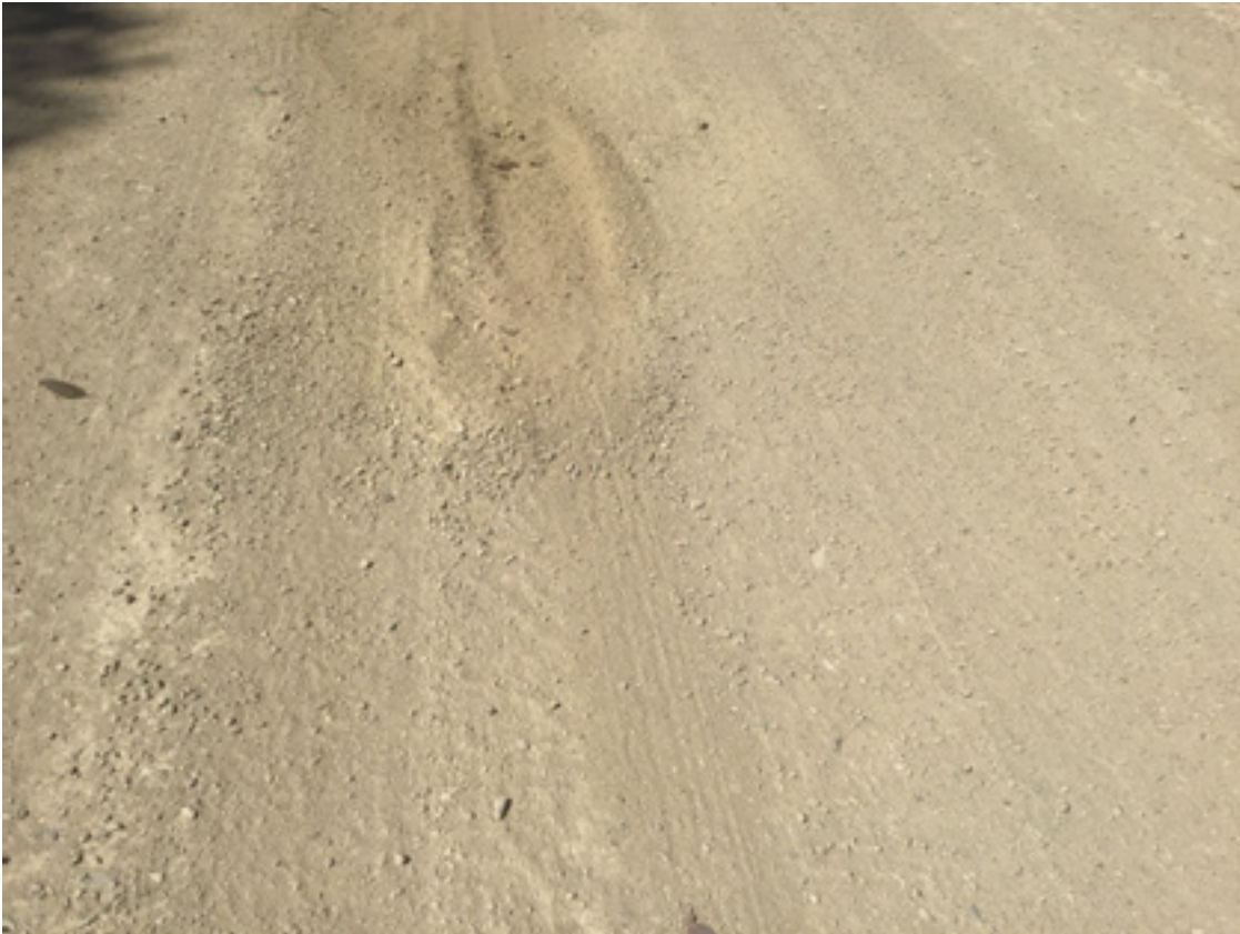
Plate 4.15 Loose material and shoving – East of Five Day Creek
