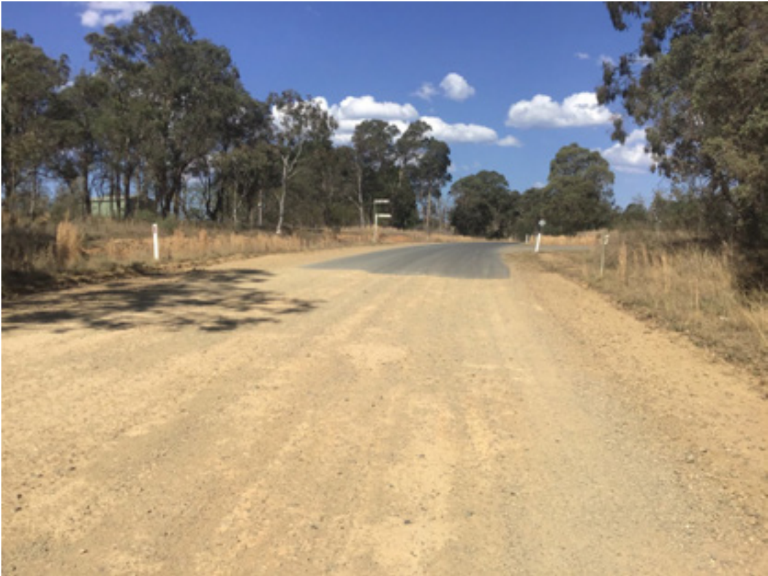
Plate 4.10 Channel erosion and potholes – North of Williams Road
