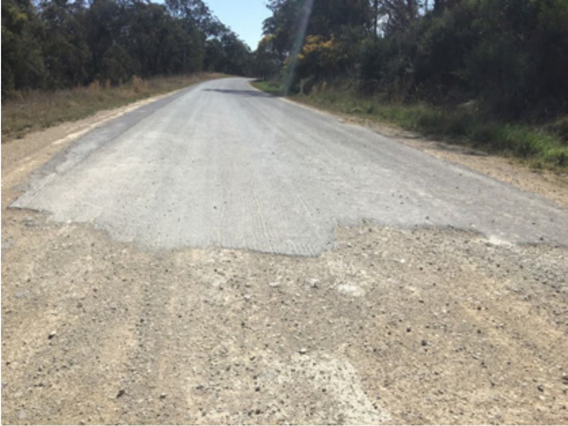
Plate 4.5 Pavement connection seam with signs of deterioration – South of Williams Road
