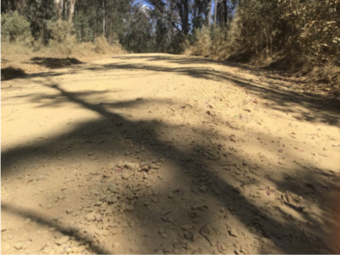
Plate 4.7 Protruding aggregates/rocks and loose materials – North of Falls Road
