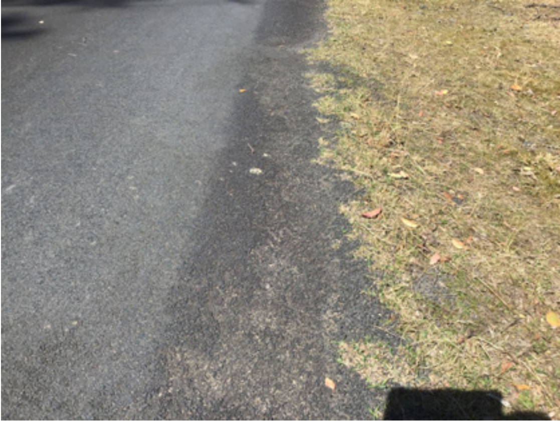
Plate 4.3 Ravelling observed on edges of seal – South of Styx River Crossing
