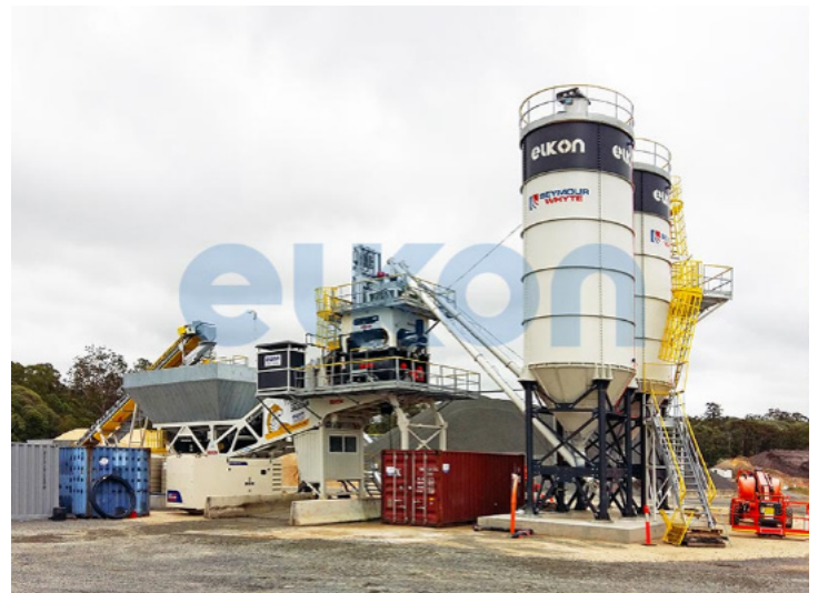
Typical batch plant facility
