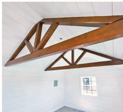
Painted ship lap siding, stained ceiling ties, breaker box, electrical package
