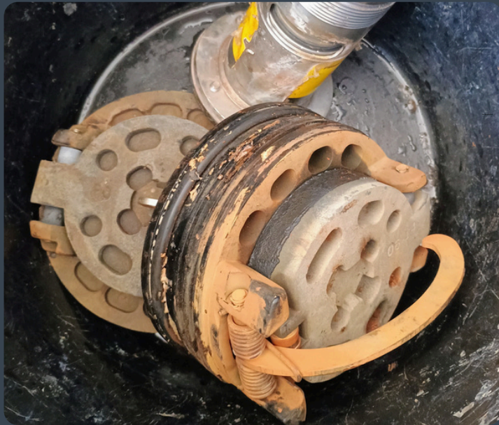
Damaged parts removed from the school's water line.
