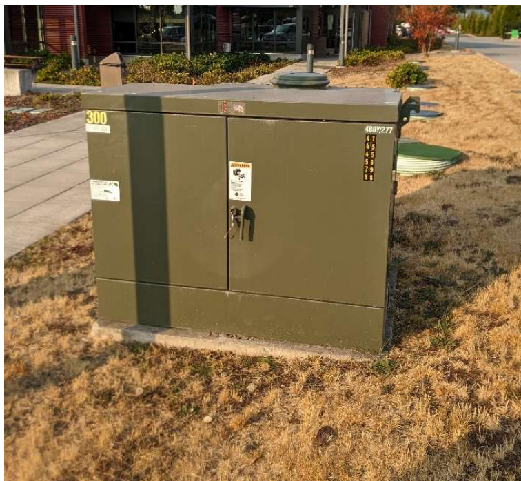
Figure 6 Whidbey Island Coupeville Facility Distribution Transformer
