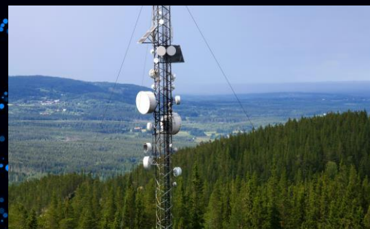
Fixed Wireless Access
