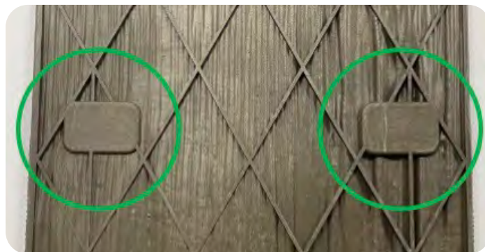
Figure 2.7.3 Fastener pads (back)
