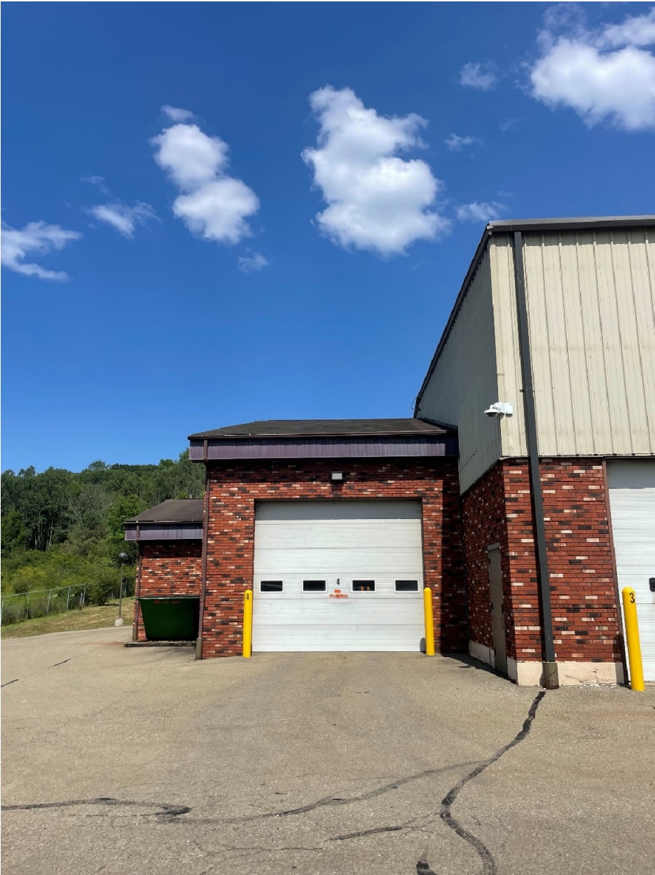
Photo of Bus Wash Roofs: To Include Main Bus Wash Roof and Addition Roof, on the Left.
