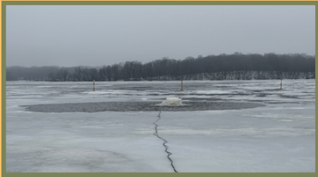
Surface aerator in Benjamin Bay, winter 2025-2026. Note the connection lines in the foreground and thin ice sign posts in the background.
