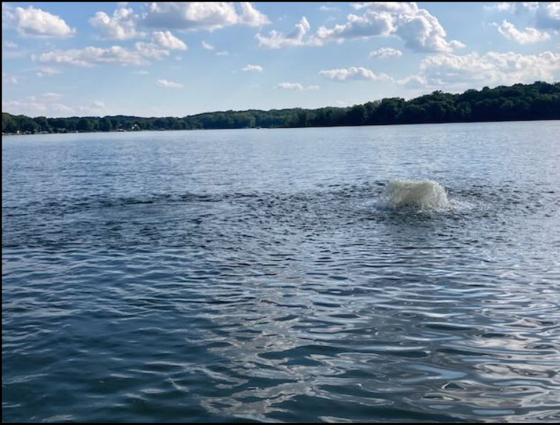
Surface Aerator/Diffuser Pair
