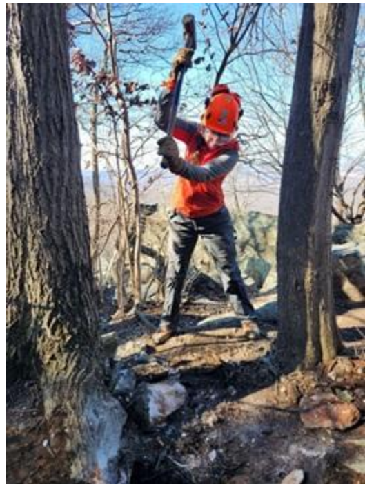
by Bill Greenan - Pictured: Janet Arici - Sometimes when a rock is in the wrong place, the best solution is to break it up instead of digging it out.
