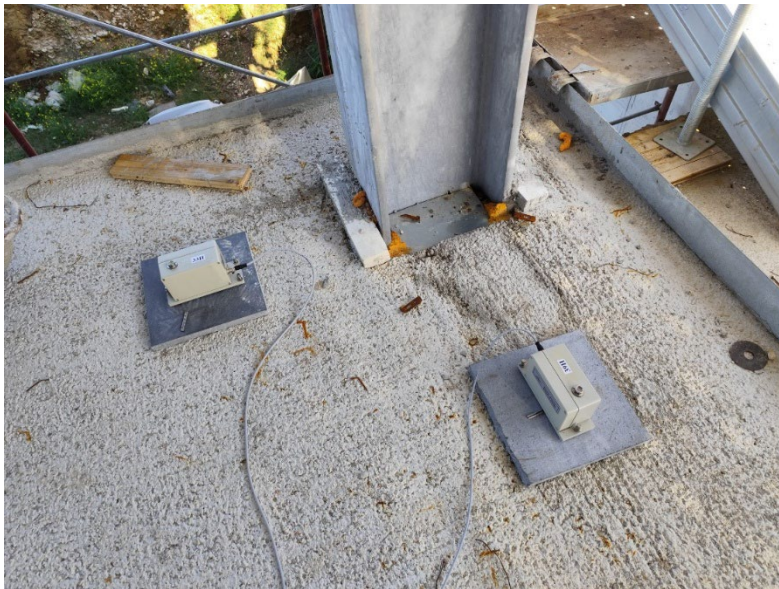
Figure 7.3: A couple of sensors placed near the corner column during the first campaign
