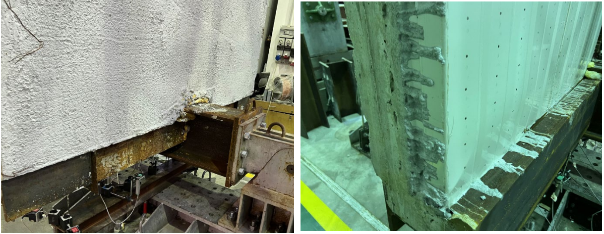
Figure 3.15: Damage patterns (negligible damage in the floor, only slight local buckling of the steel sheeting)
