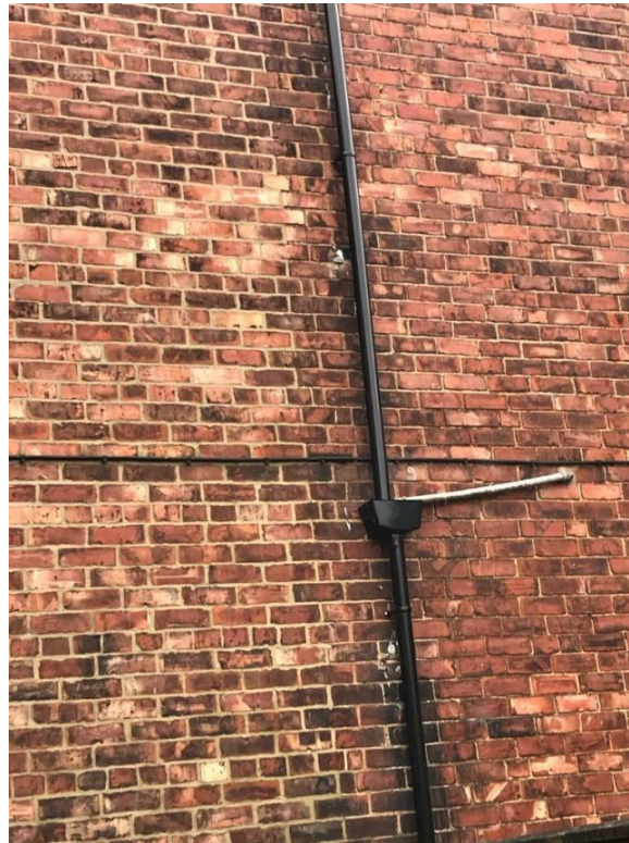
Fig 18: Note the difference in the brickwork between Number 2 (on the left) and Number 1 (on the right).
