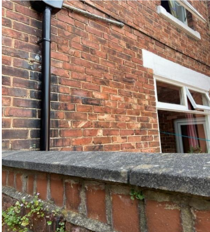
Fig 8: the picture reveals slightly different brickwork in the last section of the terrace.
