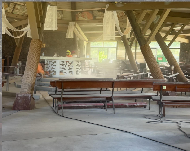
The floors of the church are also being redone due to water damages, including the sanctuary area. All carpet has been removed.
