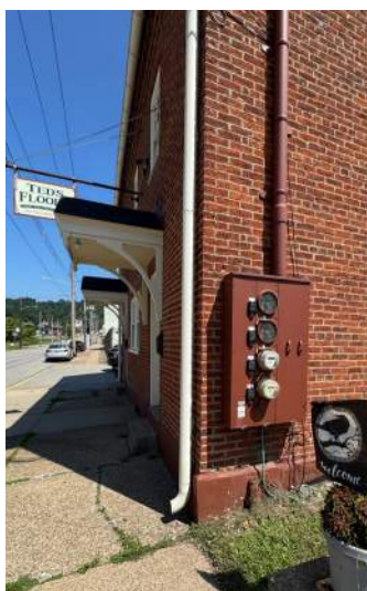
Example of a meter located on a secondary facade.
