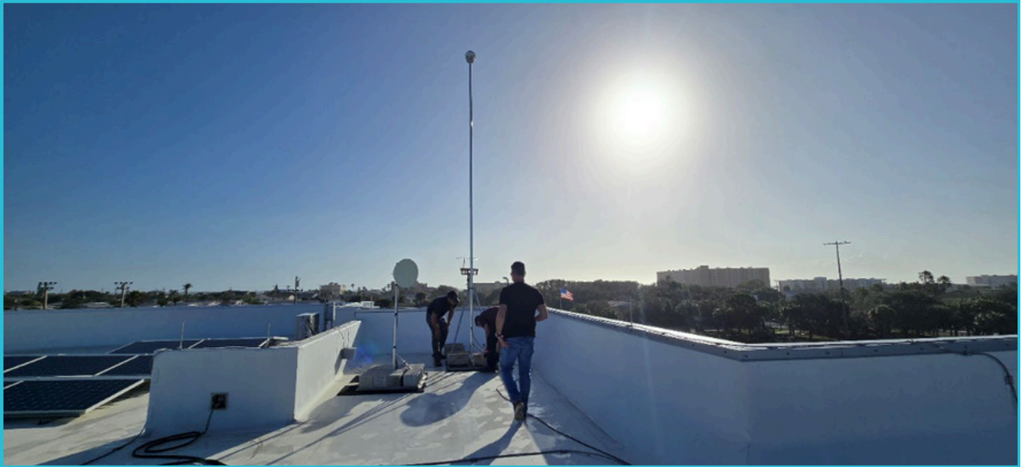
Figure 9. C5 installed CMCE-120 device.
