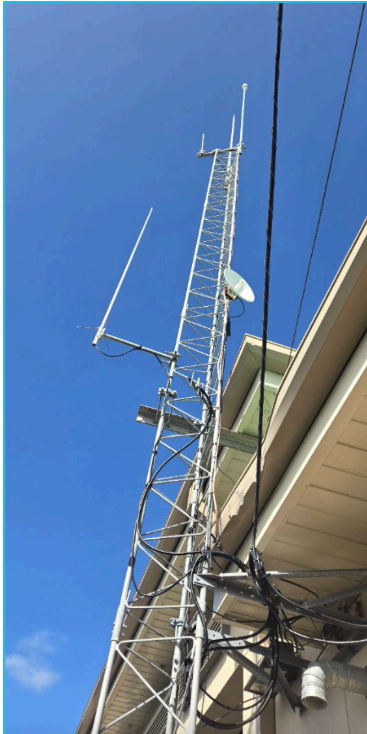
Figure 10. Installed CMCE-55 device atop Canaveral Fire Rescue Station #53.
