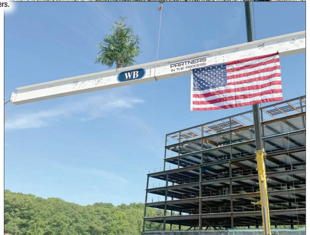
The final beam for the current phase of the Singing Bridge Residents project begins its ascent.
