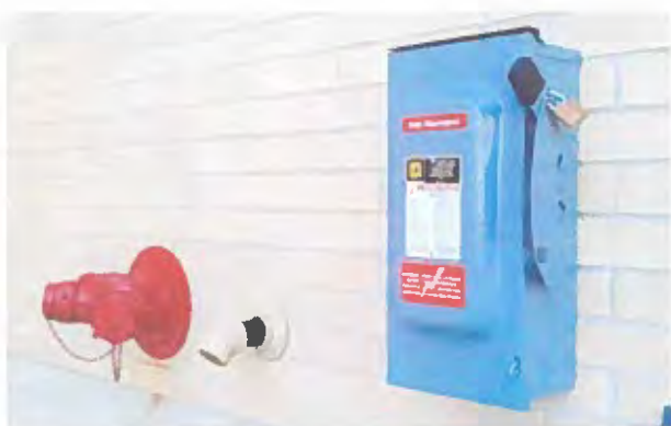
Figure 4: Utility accessible disconnect (locked in “Closed” position) installed outside next to Electric Utility Meter.
