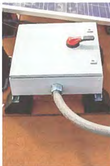
Figure 3: DC Sub-Array disconnect switch in the Open (OFF) position on a SolarBos combiner box.
