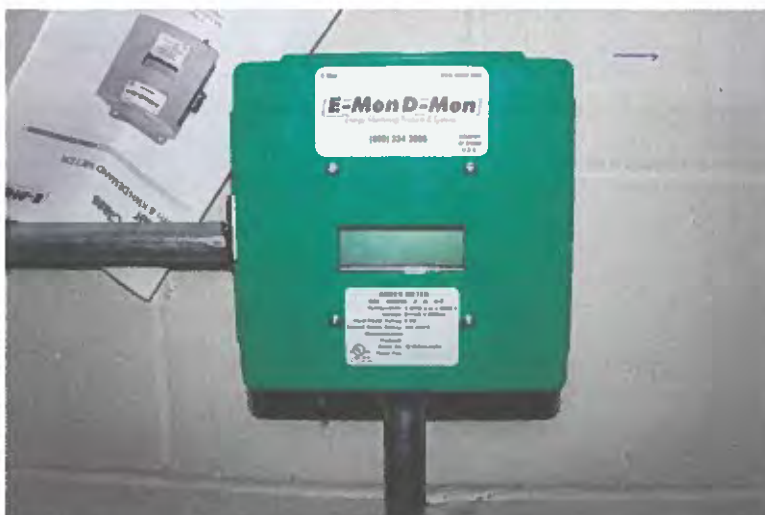
Figure 6: E-Mon D-Mon green revenue grade meter installed at MCUMTA
