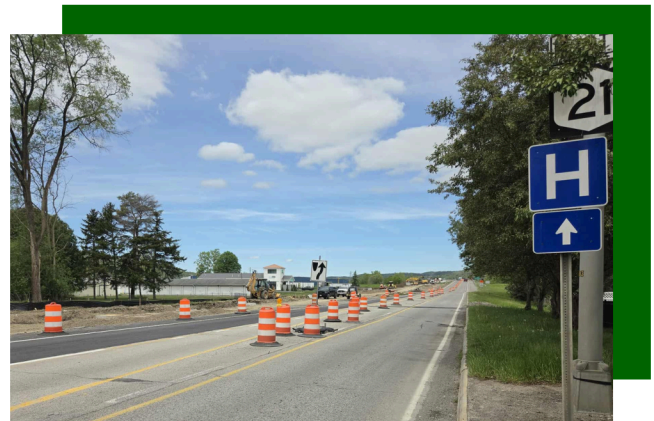
Photo (Right): Construction begins on the NYSDOT State Route 36 project from Adsit Street through Webbs Crossing, with work slated from Adsit Street through Cass Street next year. Public safety representatives offers tips for safer travel during construction.
