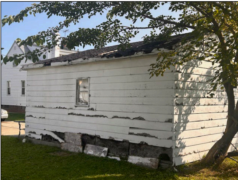
Photos 3 and 4: Garage, North Elevation and West Elevation with Tree for Removal, 23100 Ivan Avenue
