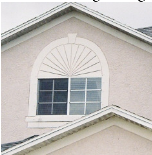
Acceptable: anchor bolts permanently attached to home
