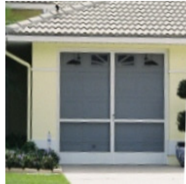
Unacceptable: screened in over garage door
