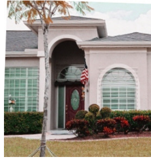
Unacceptable: plastic panels permanently attached to home.
