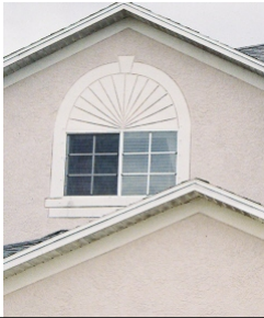
Acceptable: anchor bolts permanently attached to home
