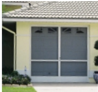
Unacceptable: screened in over garage
