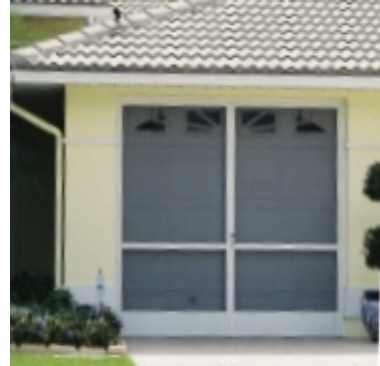
Unacceptable: screened in over garage door
