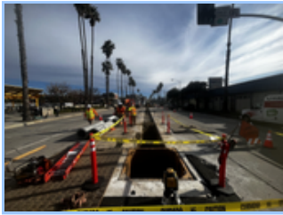
Stormwater Infrastructure on Washington Boulevard
