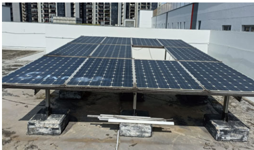
Figure 4-2 Rooftop Photovoltaics at Singapore Canadian International School
