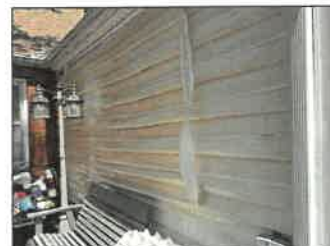
The siding melted—if it had gone through, the house would have burned.
