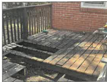
The firemen had to remove part of my deck to make sure the house was not on fire.
