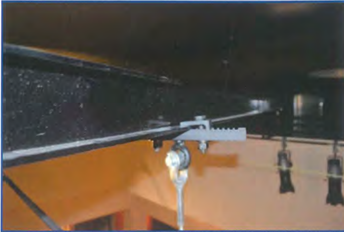
Cables fastened with a swaged socket to beam clamps on gantry beam
