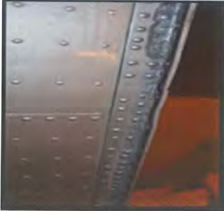
Attachment flange damage
