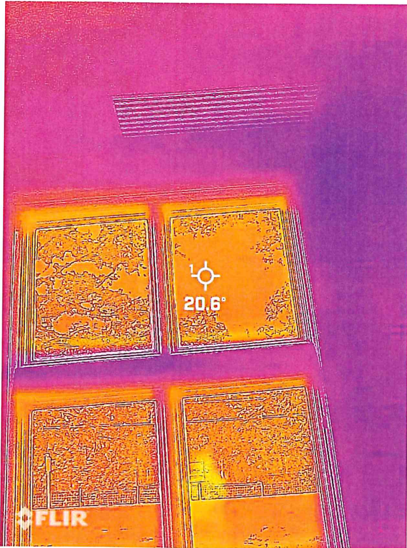
35 49-East Inside 3 above window Date Taken: 6/18/2026
