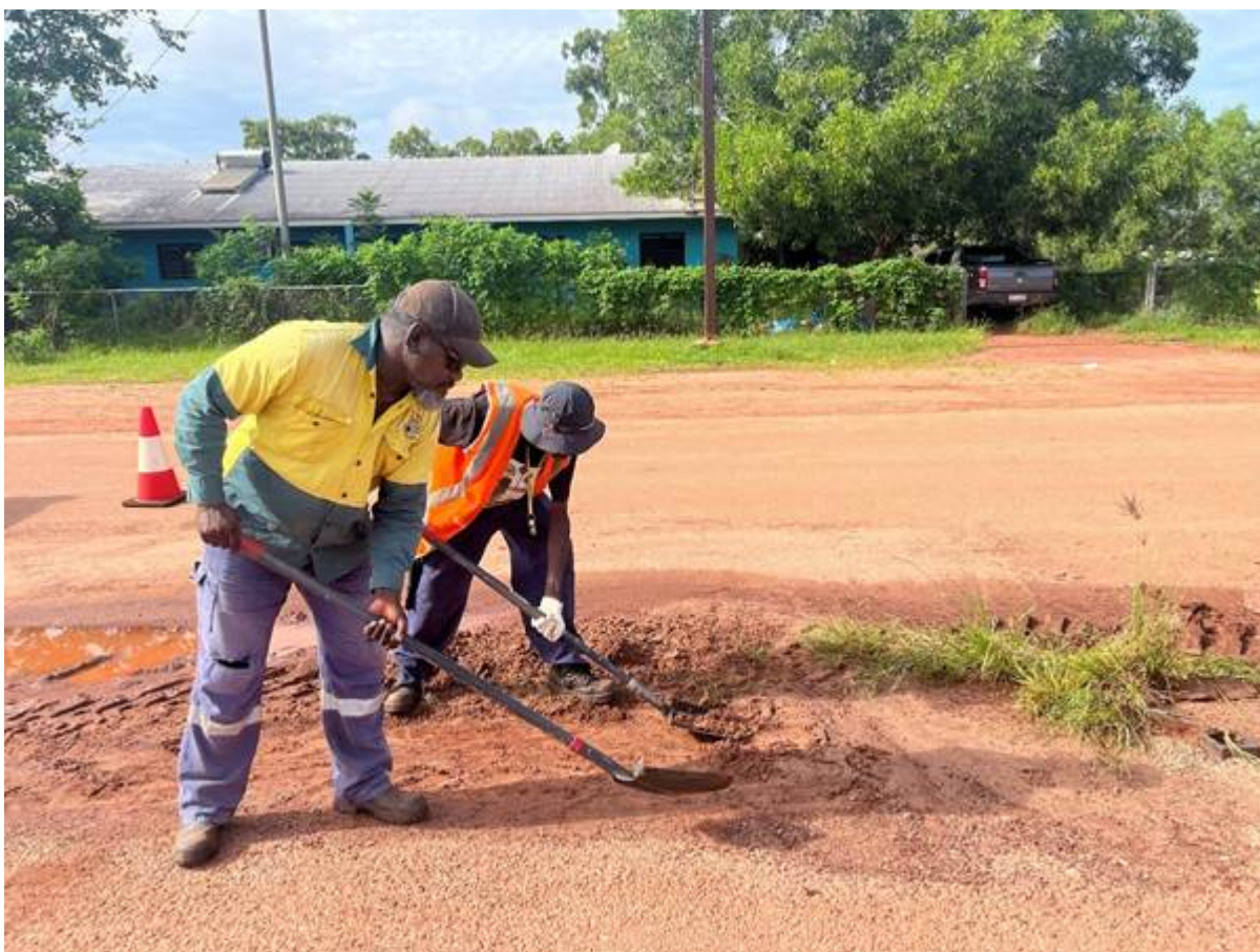
Municipal Services Officers James Wunungmurra and Daniel Gumbula carrying out maintenance work in the Gapuwiyak community
