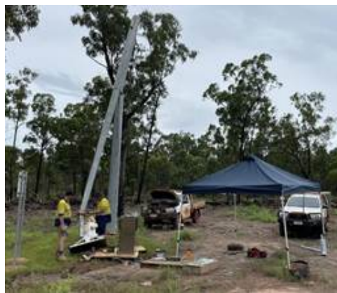
CCTV installation November 2025 Galiwinku
